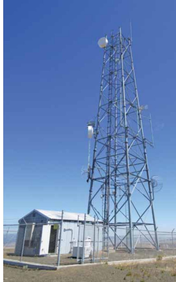
Juniper Point upgraded radio site
